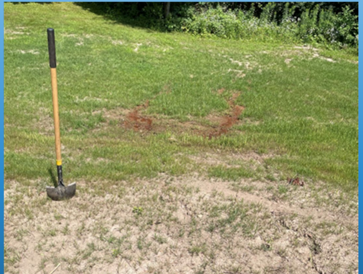
This is a recently installed but failed mound system. The soil was compacted and could not infiltrate the wastewater. This led to the system discharging wastewater to grade on the downslope side, or what is commonly called a "leaky toe."
