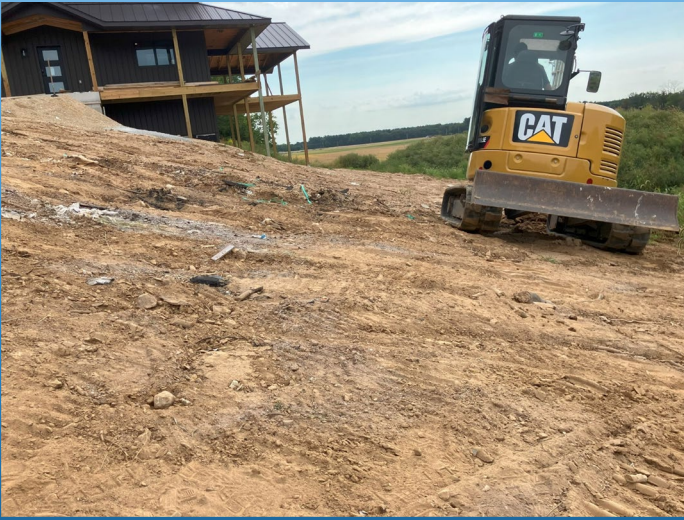
This is the area where an at-grade system was planned. Due to the grading, a new site had to be found, a new soil test conducted, and a new design proposed.
