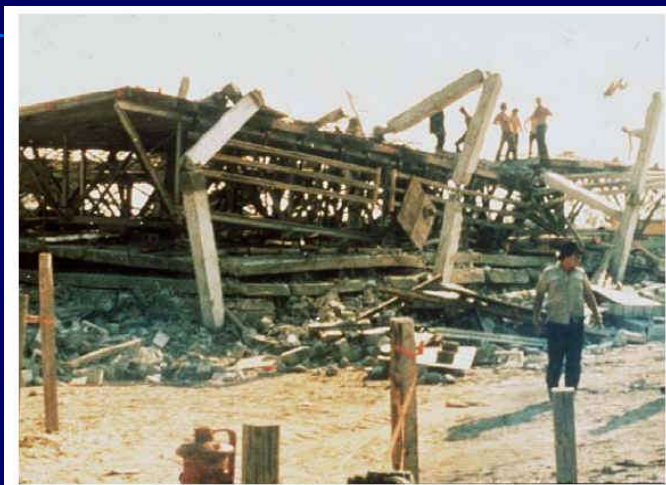
5-8a: Harbour Cay Condominium collapse (NBS/NIST)
