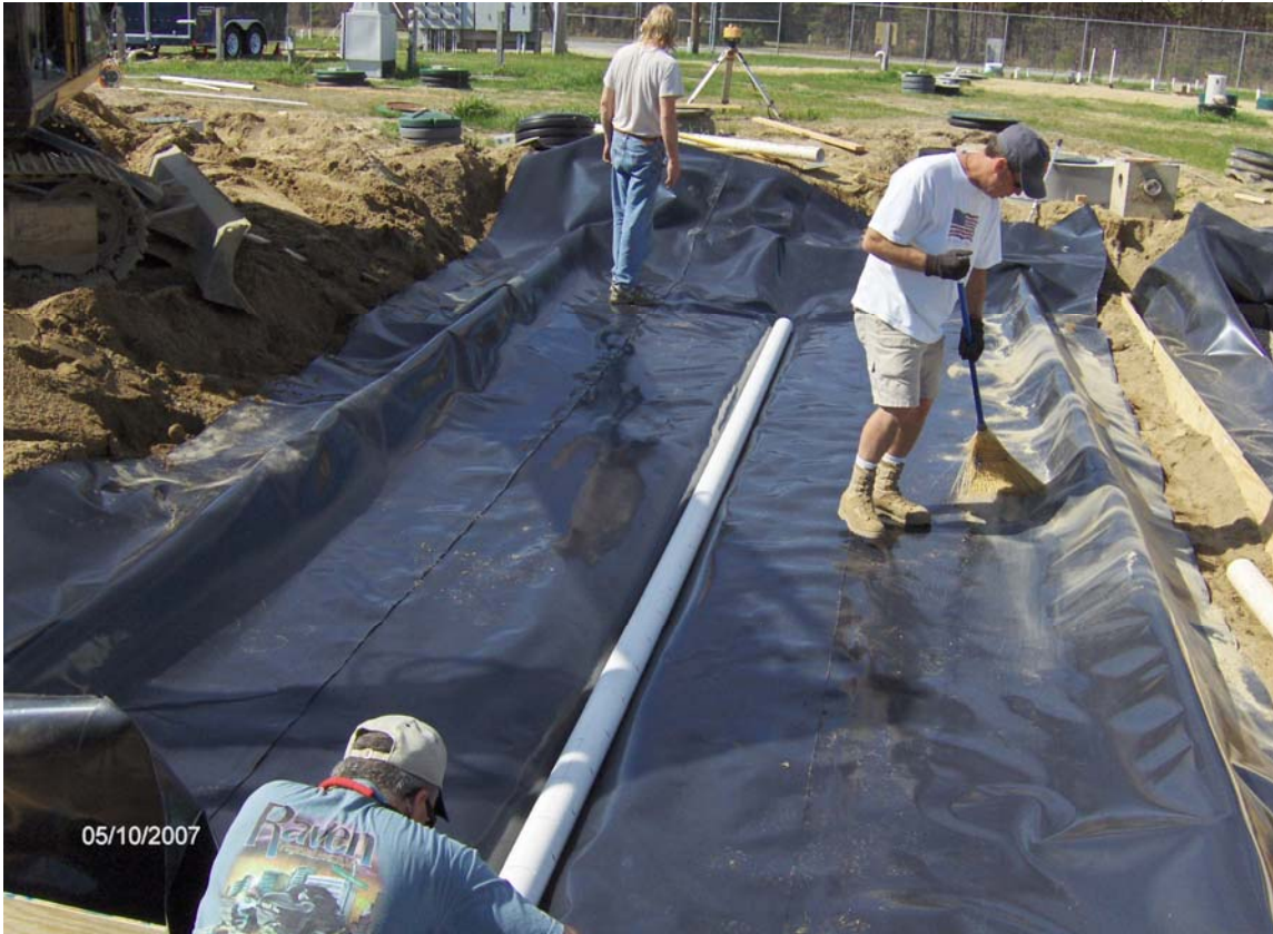
Figure 1. A wooden frame was constructed to hold an impervious liner in place. The ground beneath the liner was prepared to slope toward the center collection drain. A groove in the supporting soil was installed and sloped toward the sampling point.
