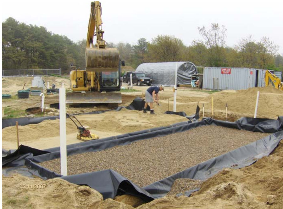
Figure 4. Twelve inches of sand are placed over the 1/8 inch aggregate (left-hand cell), compacted in six-inch lifts. The right-hand cell is ready for initial sand placement. The prepared sand area is leveled and readied for the placement of the Eljen GSF modules.
