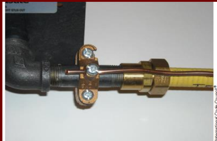
Bonding of CSST gas piping
