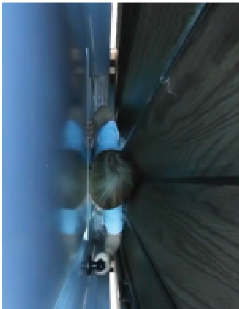
A four-year-old child in the space with the landing door and elevator door closed
