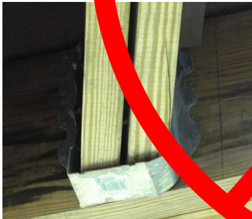
Wrong hanger type
