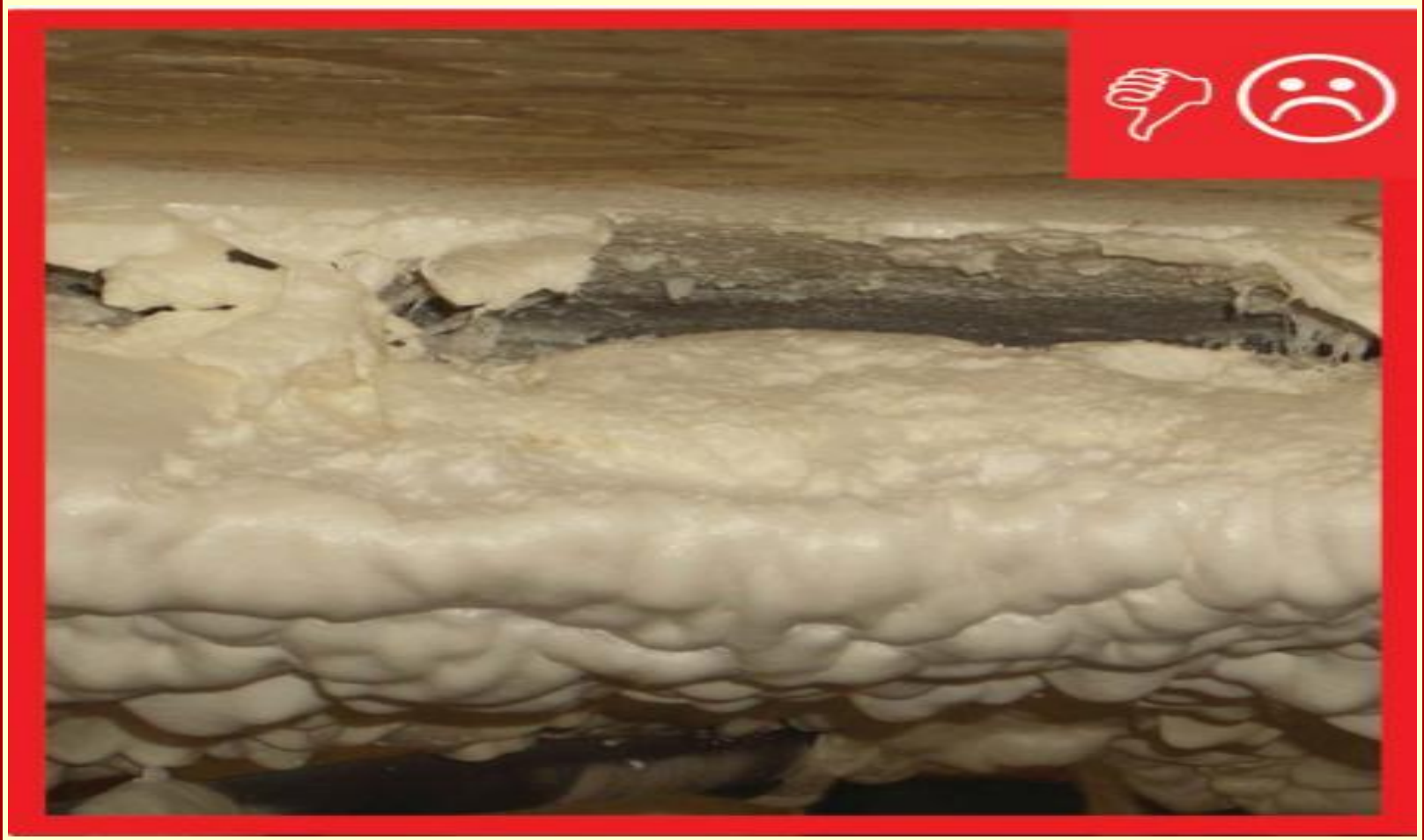
Spray foam installed with voids
